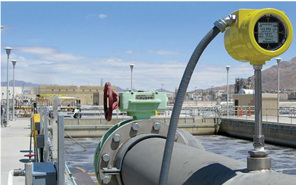
Figure 5. In outdoor, harsh desert sunlight, know the ambient conditions of your installation location.
