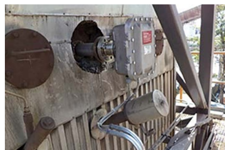
Figure 3A Top: Small diameter piping situations can require a different type of connection configuration.
